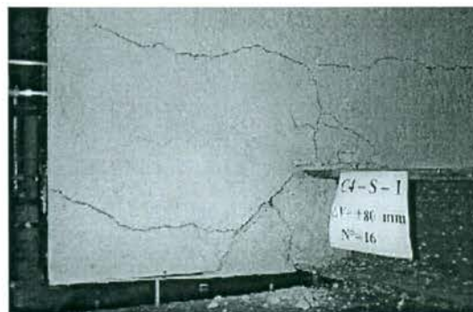
Figure 4: Damage in the concrete slab
