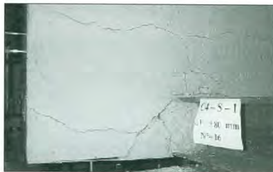
Fig. 5 Damage in the concrete slab.
