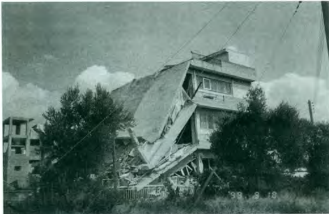
11 – Athens (1999) earthquake. Collapse of a part of a r.c. building. Note unbroken glasses of the intact portion of the building.
