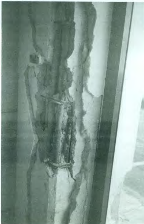
3b – Athens (1999) earthquake. Details of damage at midheight of columns, bars buckled.
