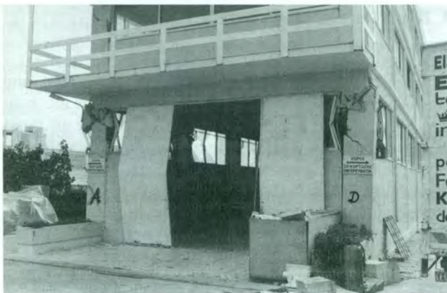
8a – Athens (1999) earthquake. Compression damage at the base columns of a warehouse. Note the symmetrical buckling of bars and of window frames.
