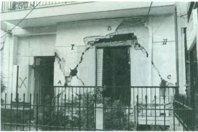
6a – Athens (1999) earthquake. Damage to partitions at ground level. There is a very poor evidence of lateral displacements.
