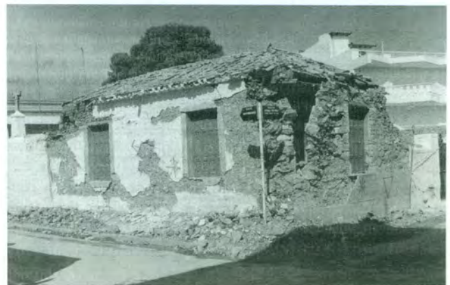
9 – Athens (1999) earthquake. Symmetrical compression damage to a masonry building.
