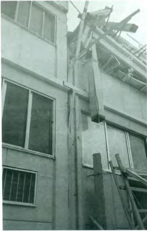
10 – Athens (1999) earthquake. Upper storey compression failure. No evidence of lateral displacements.
