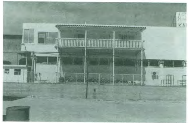
4 – Athens (1999) earthquake. Compression damage to short columns. Note the symmetrical buckling of window frames.
