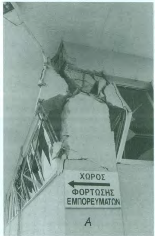
8b – Athens (1999) earthquake. Details of damage of fig. 8a.
