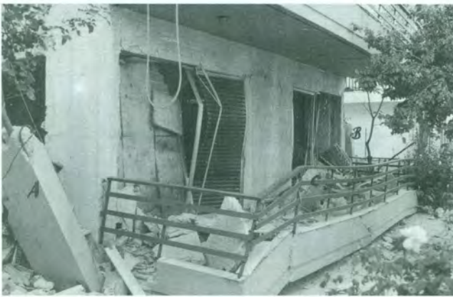
7 – Athens (1999) earthquake. Columns of the collapsed open ground floor penetrated almost symmetrically the slab of the first storey.
