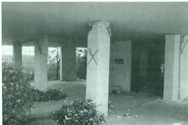
2a – Athens (1999) earthquake. Interior columns of a modern r.c. building. There is a poor evidence of lateral motion.
