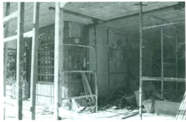
2b – Athens (1999) earthquake. Damage at the ground floor. Glasses are intact.
