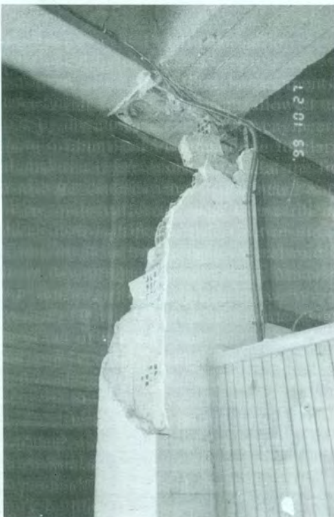
5e – Compression damage to brick masonry column. Note the unbroken window.
