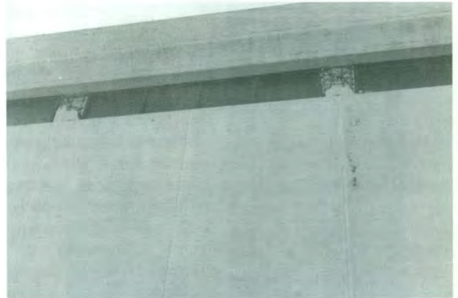
5b – Athens (1999) earthquake. Details of damage to short columns.
