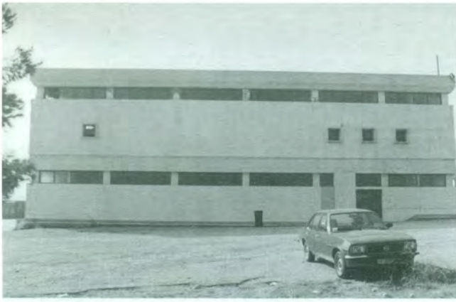
5a – Athens (1999) earthquake. Compression damage to short columns. Glasses are intact. There is no evidence of lateral displacements.
