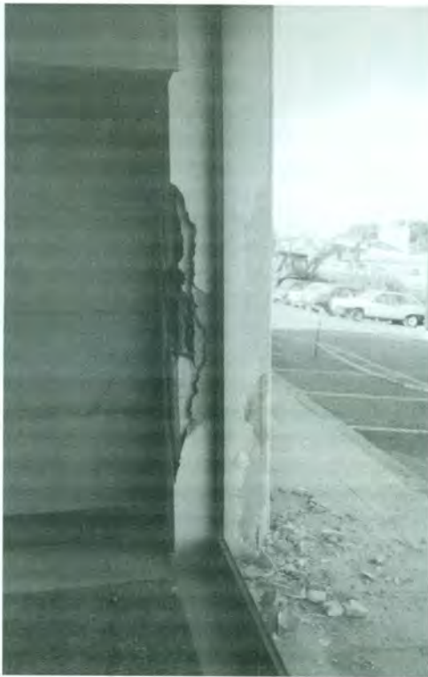
3a – Athens (1999) earthquake. Damage at midheight of columns.
