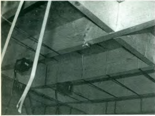
Picture 4 – Ceiling of the first storey. The two accelerometers are shown attached to the main beams. Some of the plastic ribbons tightening the loading sacks with the sand, were broken after a number of tests. One wooden beam was broken after the 20th repetition of the earthquake.
