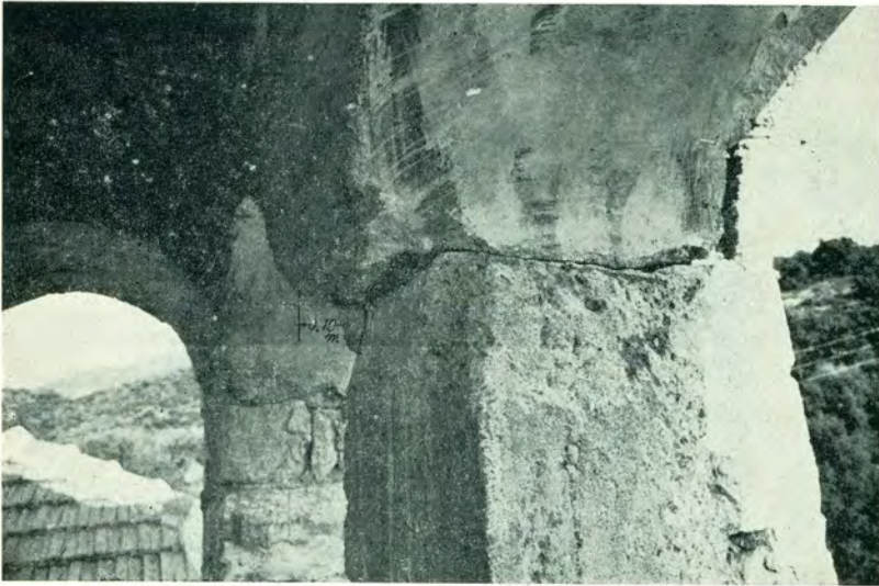
Fig. 29. Construction joint with no connection of the two adjacent parts, caused a dislocation of the top part of the church steeple at Kaloudi.
